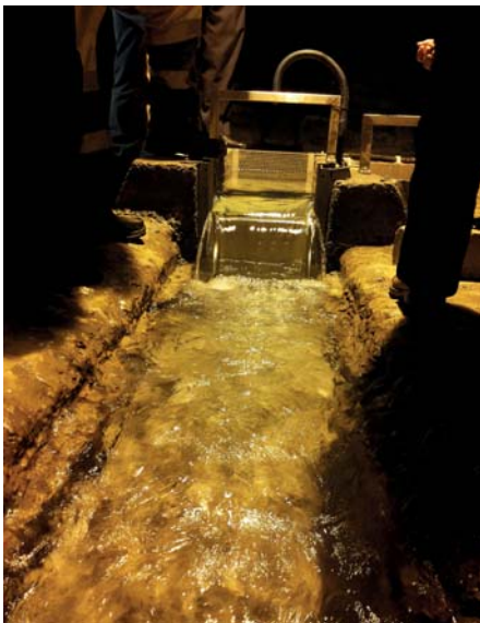
Figure 2. Automated rectangular weir measuring seepage flow inside Komani dam.
